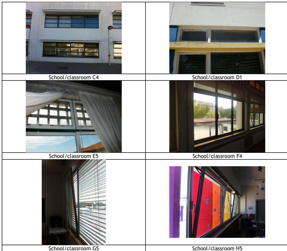
Figure 2 - Photographs showing windows opening mode selected for ventilation during test of airborne sound insulation of classrooms façades.
