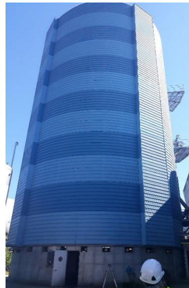
Figure 8. Anaerobic digester for biodegradable wastes.
