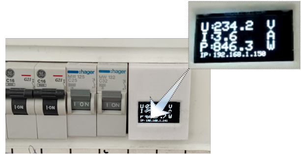
Fig. 2. Consumption monitor hardware/Energy Meter
