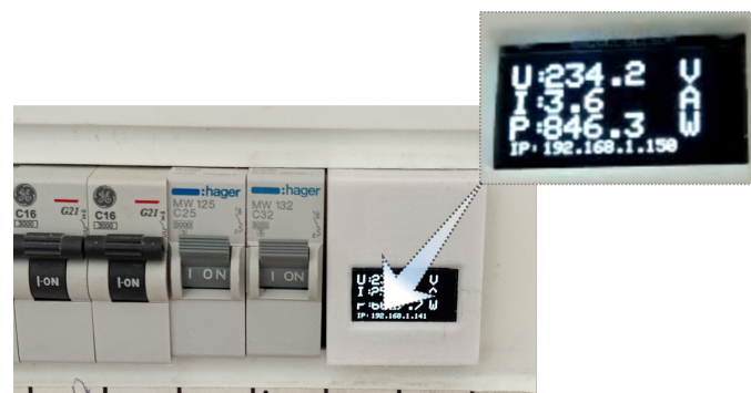
Figure 12: Consumption monitor hardware/Energy Meter
