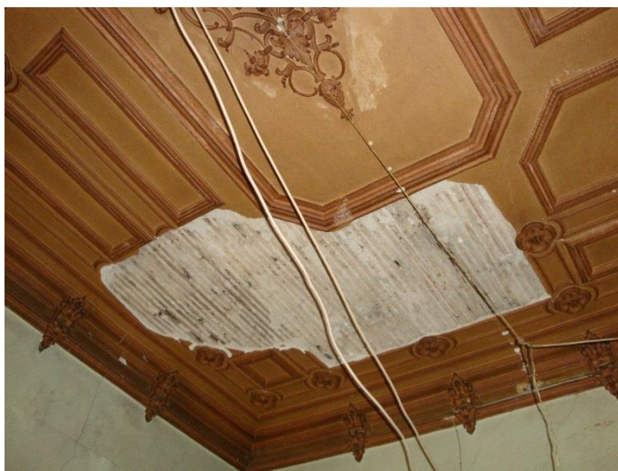
Figura 2.46: Descasque do reboco
